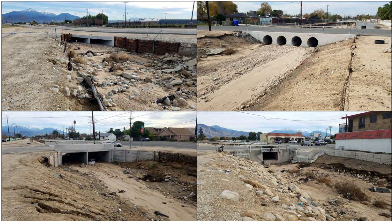
Figure 9. Typical bridges and culverts along the City Creek Channel. Clockwise from upper left: Third Street crossing, view to the east; Del Rosa Avenue crossing, view to the southwest; Tippecanoe Avenue crossing, view to the east; Pedley Road crossing, view to the southeast. (Photographs taken on December 10, 2019)
