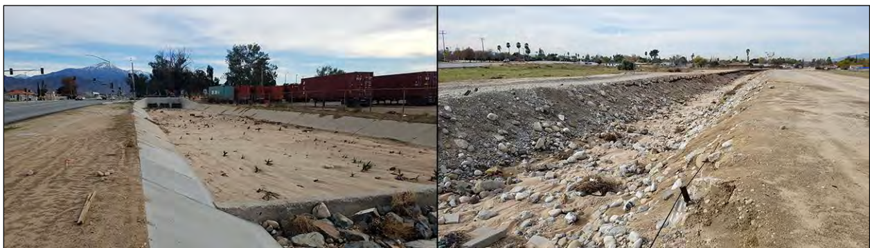
Figure 4. Current conditions of the City Creek Channel. Left : concrete-lined channel near Victoria Avenue, view to the east; right : earthen channel in the middle portion, view to the west. (Photographs taken on December 10, 2019)
